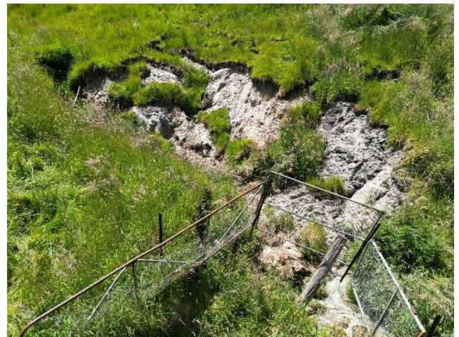
Figure 1. The lateral headcut formed and was starting to accelerate up the catchment. The fence is where the creek is fenced off and the headcut has moved up the flow line beyond the fence
