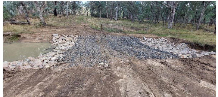
Figure 3 – this structure has a double benefit of being a grade control (slowing flow and trapping sediment above) and providing stable, long lasting access across the creek.
